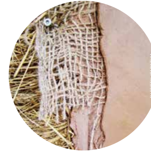
↑ A mix of clay and straw fills in the prefab timber structure.
